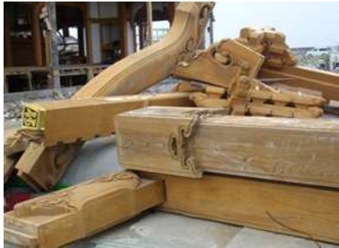
Large temple / shrine posts and beams splintered
